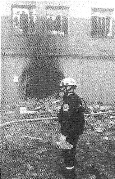
Figure 54: The round C-Ring exit hole some twelve feet across made by whatever struck the Pentagon.
