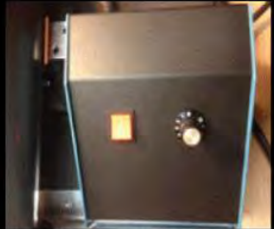
MOTOR CONTROL BOX
