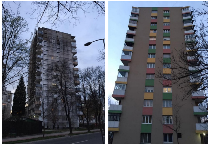
Figure 1: Appearance of one of the analyzed buildings during and after the completion of the thermal insulation procedure. Retrieved from https://www.skyscrapercity.com/threads/zenica-%D0%97%D0%B5%D0%BD%D0%B8%D1%86%D0%Bo-development-news-2020.2234552/page-4 .
