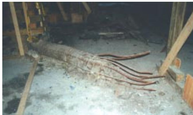
Figure 5.23 Severed column 5H
