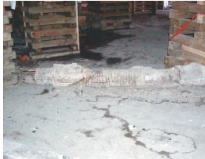
Figure 7.5a Column impacted and torn off at supports
