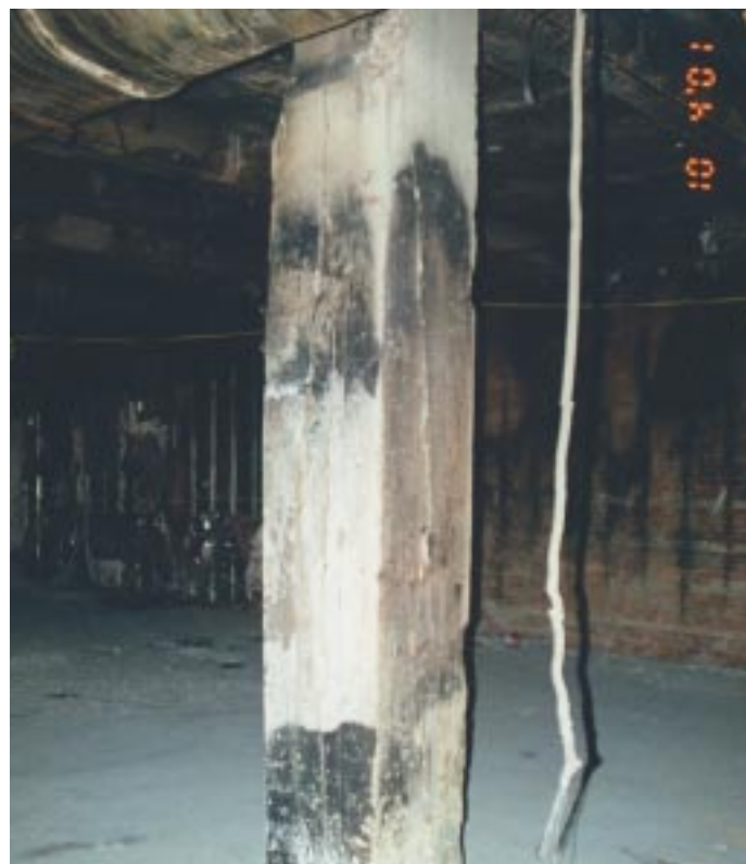
Figure 5.24 Cracked column 5N
