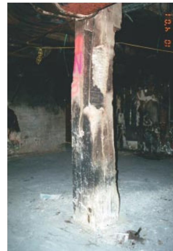
Figure 5.19 Column 3N damaged by impact and fire
