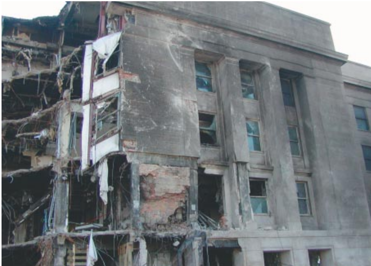
Figure 5.11 Debris scars at upper levels south of impact area
