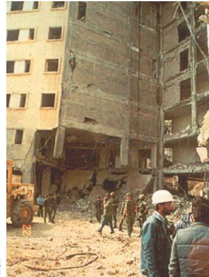
Figure 7.7 Reinforced-concrete frame with masonry filler walls acting as a vertical diaphragm to compensate for column loss
