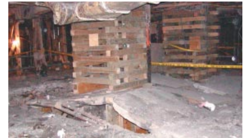
Figure 5.27 Breached second-floor slab
