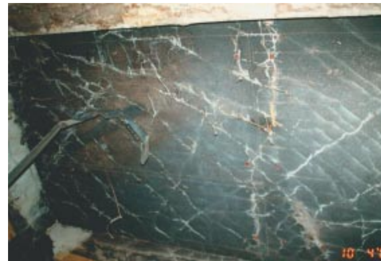
Figure 5.28 Crack patterns in second-floor slab
