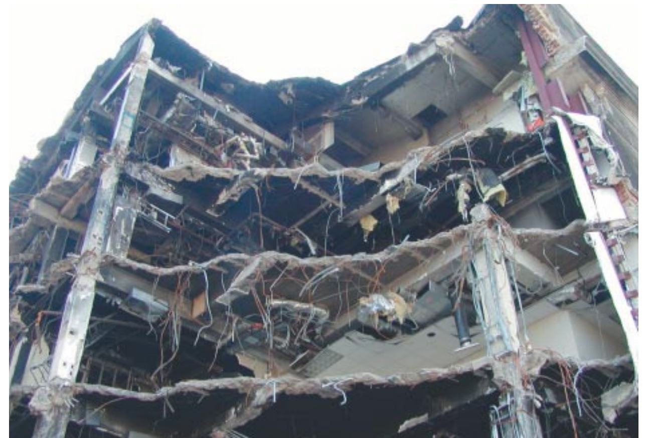
Figure 5.4 Remaining structure at southern extreme of collapse area
