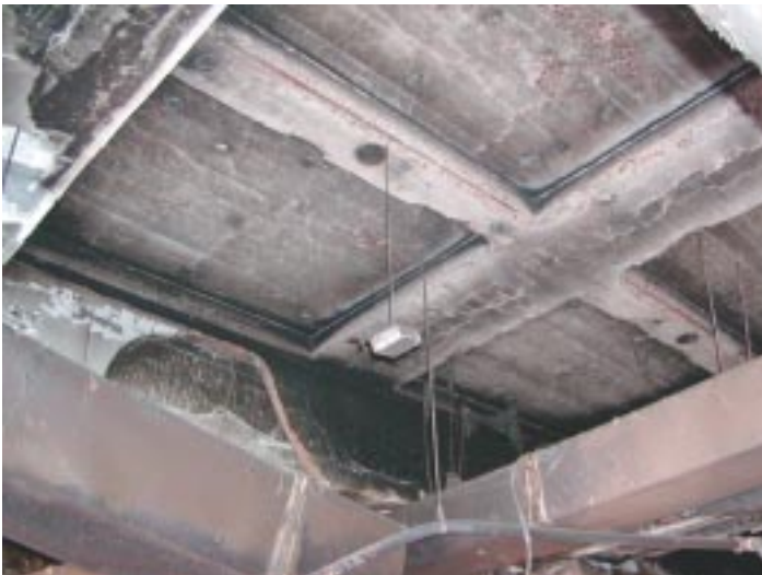
Figure 6.12 Fire damage to third-floor (light well) beams
