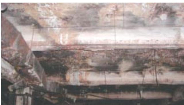
Figure 5.25 Impact and fire damage near column line C
