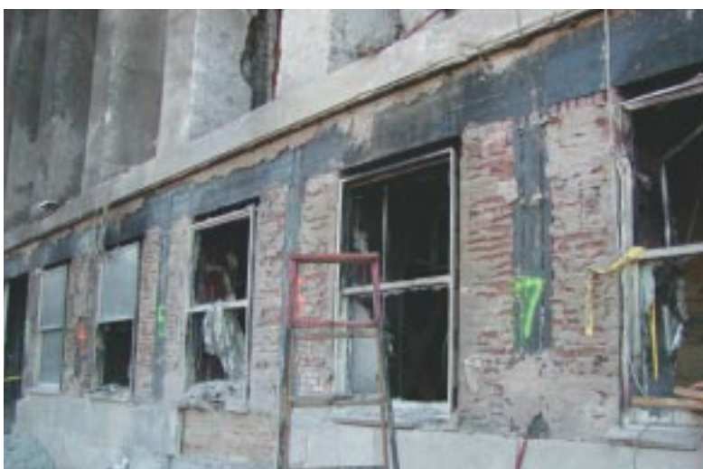
Figure 5.7 First-floor facade damage to the north of the impact area
