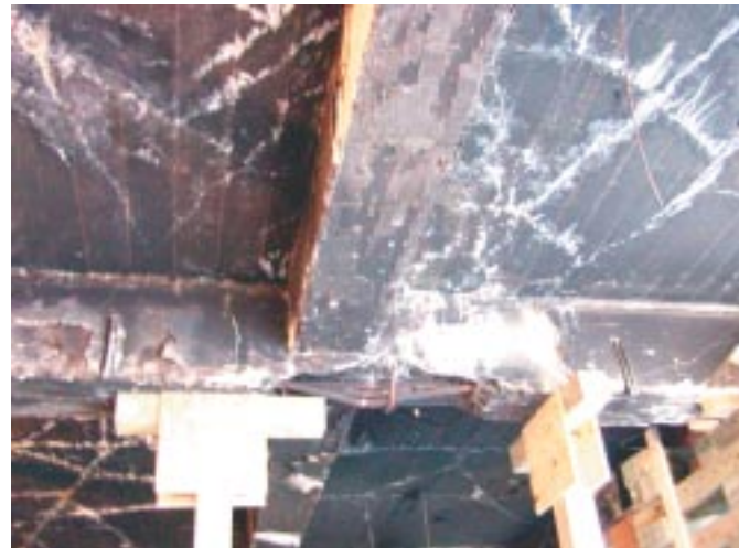
Figure 6.14 Fire-damaged second-floor beams
