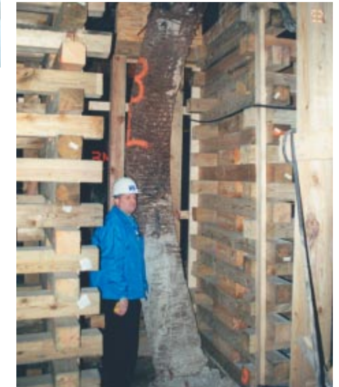
Figure 5.20 Column 3L with large deformation and discrete hinges
