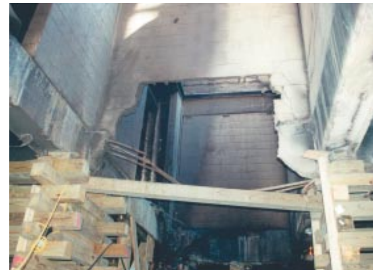
Figure 5.30 Missing beam in air shaft
