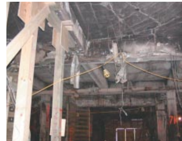
Figure 5.26 Impact damage near column 6K
