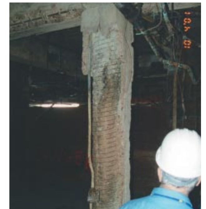
Figure 5.31 Fire damage to column in second story
