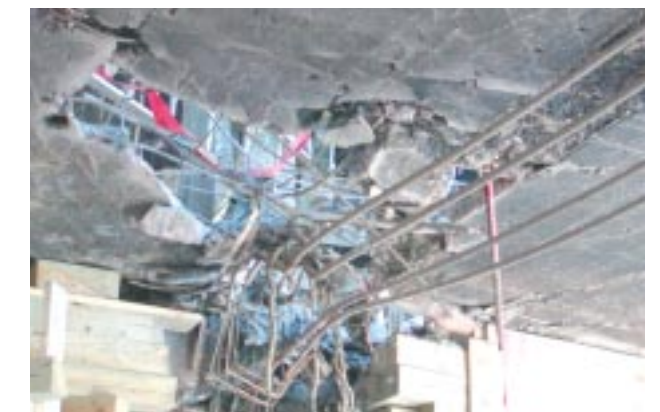
Figure 5.29 Concrete stripped from floor beam
