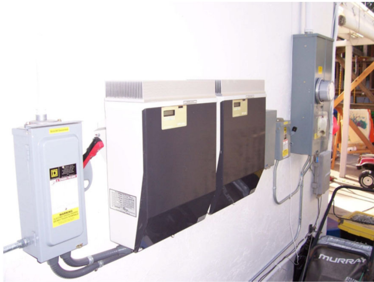
AC & DC Discos on either side of inverter – OK!
