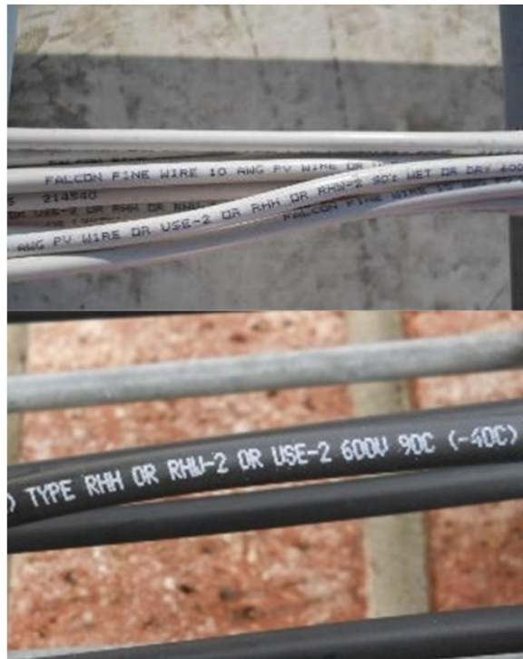
USE-2 & PV Wire outside, exposed to UV – OK!
