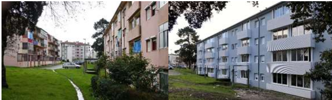
Figure 86. Cerco do Porto under refurbishment: before and after. Source: J. Restivo archive (2017); V. Moutinho archive (2018)
