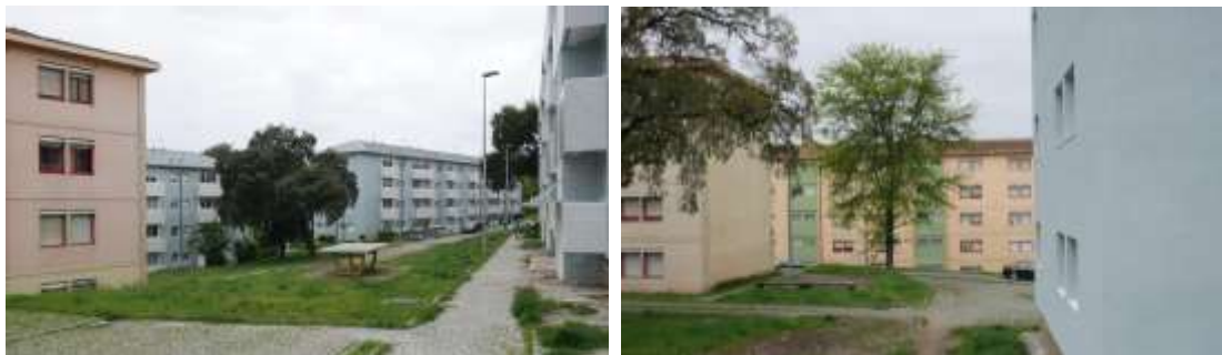
Figure 20. Cerco do Porto municipal housing, Campanhã, Porto. Both pictures: on the left side the original buildings (refurbished in the late 1990s), and on the right side the buildings under refurbishment. Source: Domus Social / J. Restivo archive (2019)
