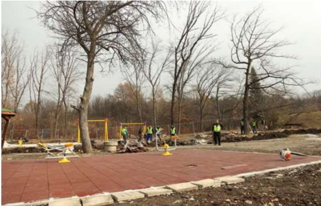
Figure 422. Public works during the second stage of the Northern parks's reconstruction, Source: http://so-nadejda.com/gallery/Other/severen-park-ul-narodni-buditeli-sche-bde-obnoven-do-kraya-na-2019-g/126.html
