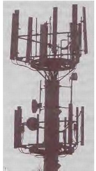
Figure 237: This little lot is right next to a public swimming pool and sports centre
